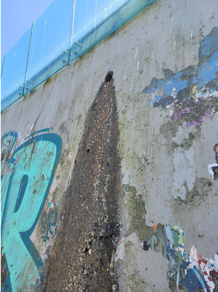
Figure 5: An image of a drainage pipe from the residential homes that run along the length of the beach.
